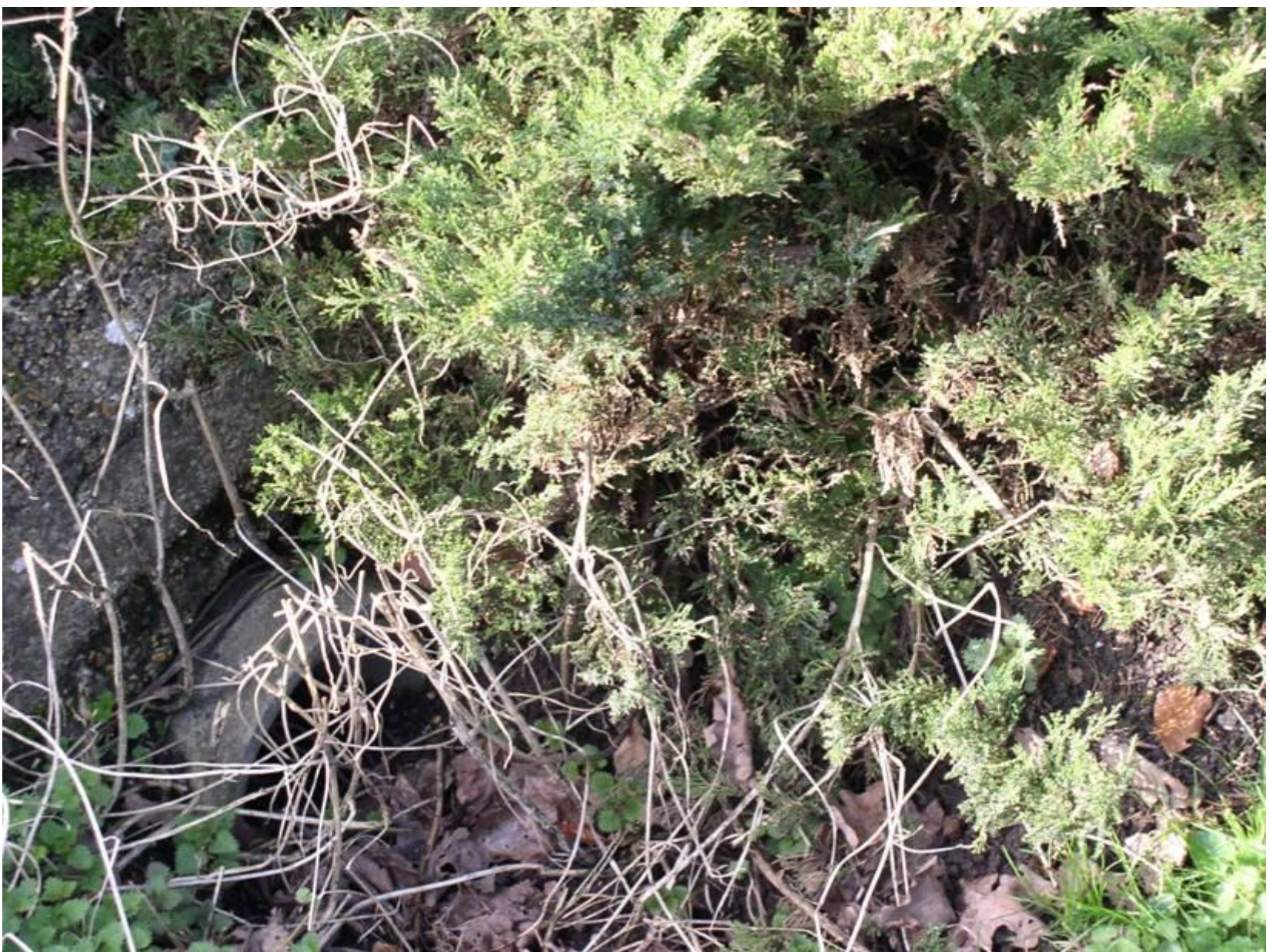
South east end of the culvert for the entrance to Trin's Close. This again shows that the ditch needs digging out.
