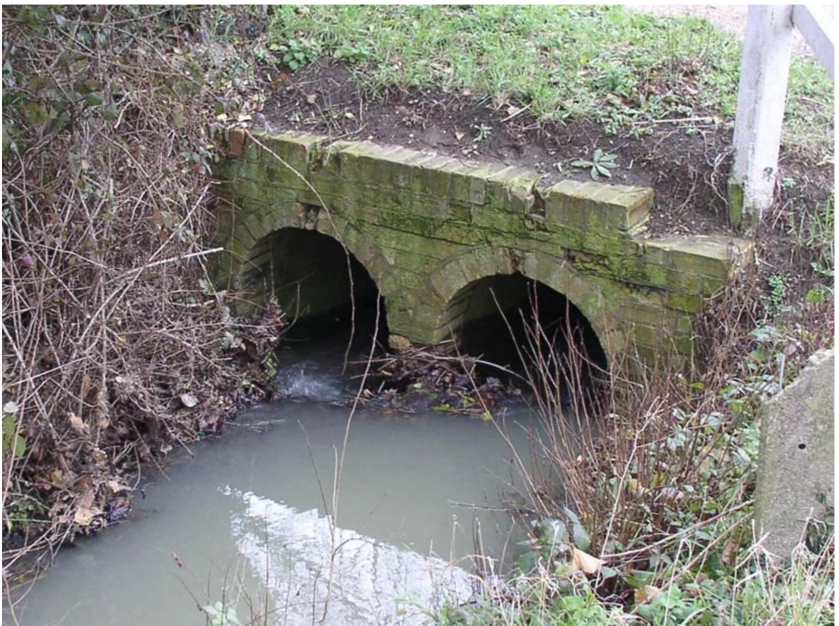
Build-up of natural debris at the culvert at Green End House. This was causing some backing up of the water.
