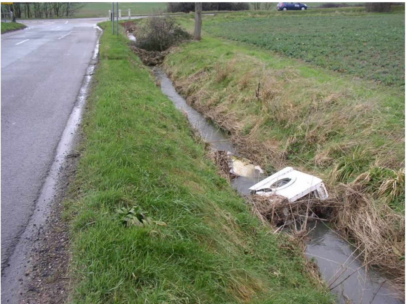
Potential blockage from discarded washing machine just east of B1040/Rogue's Lane junction.
