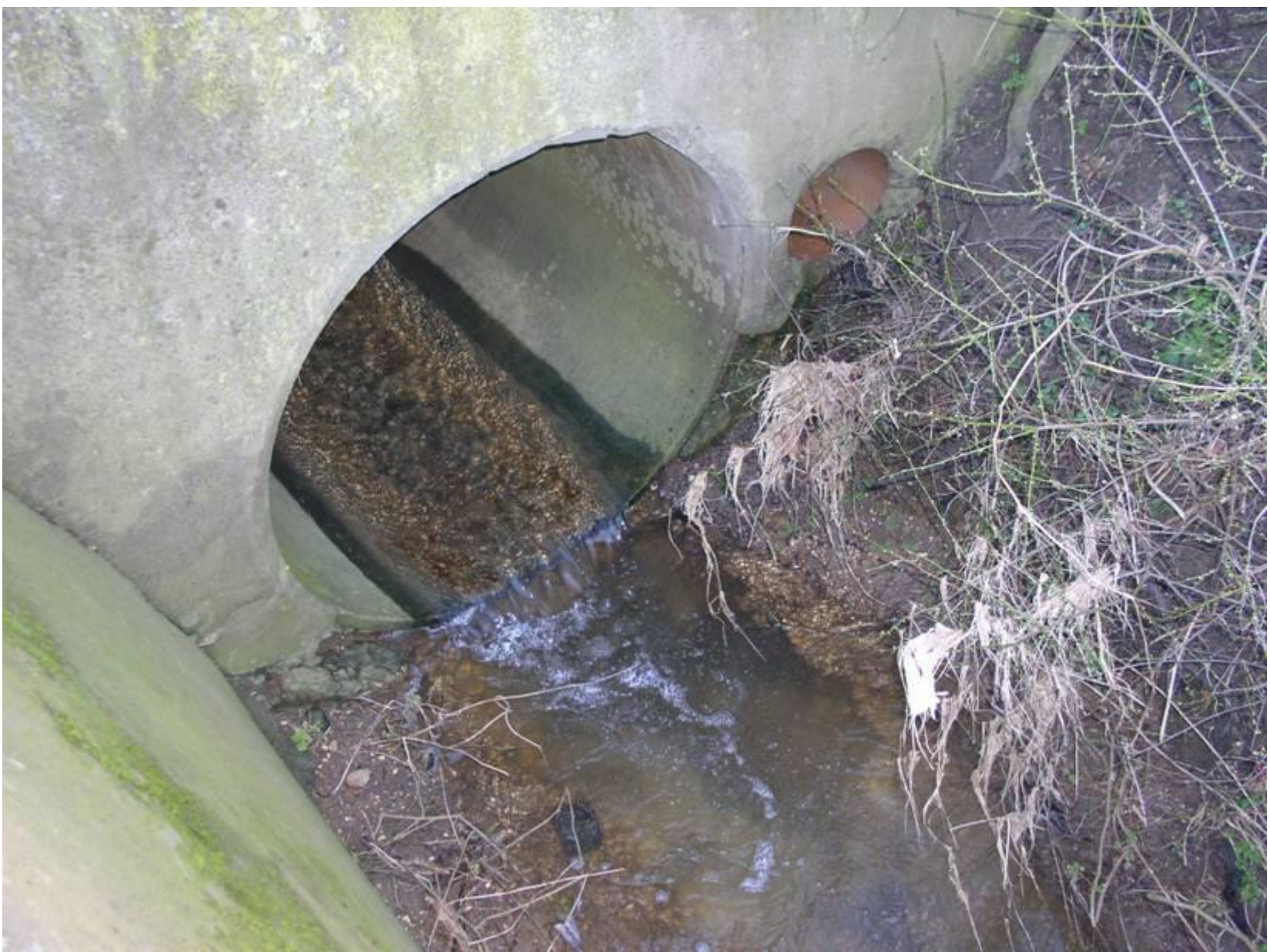
South-eastern end of the culvert where the Fentstanton Road crosses the Main Drain near the chicken farm. This has been dug out to too great a depth by HDC.
