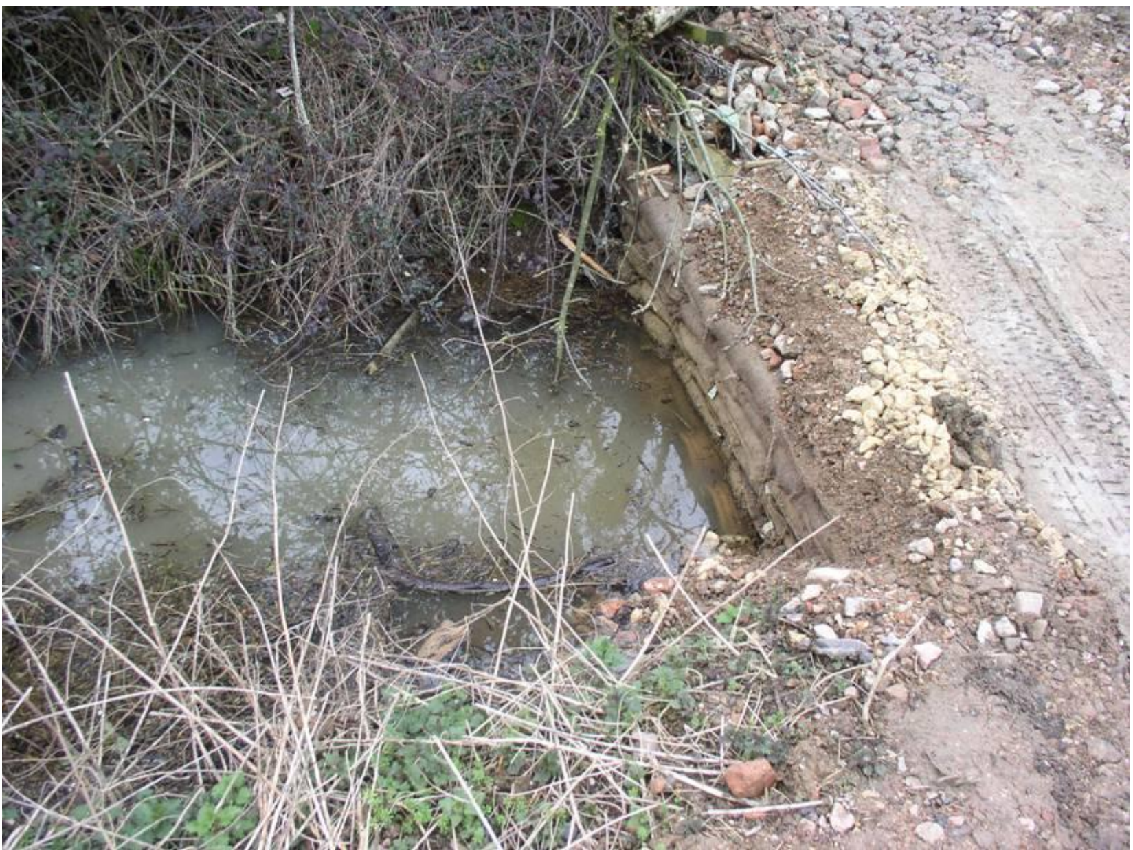
Standing water unable to drain away at the entrance to the building site opposite Hilton Hall. The owner of Hilton Hall finds that when water remains in this ditch for a period of time without draining, then it causes damp in his 'cellar'.
