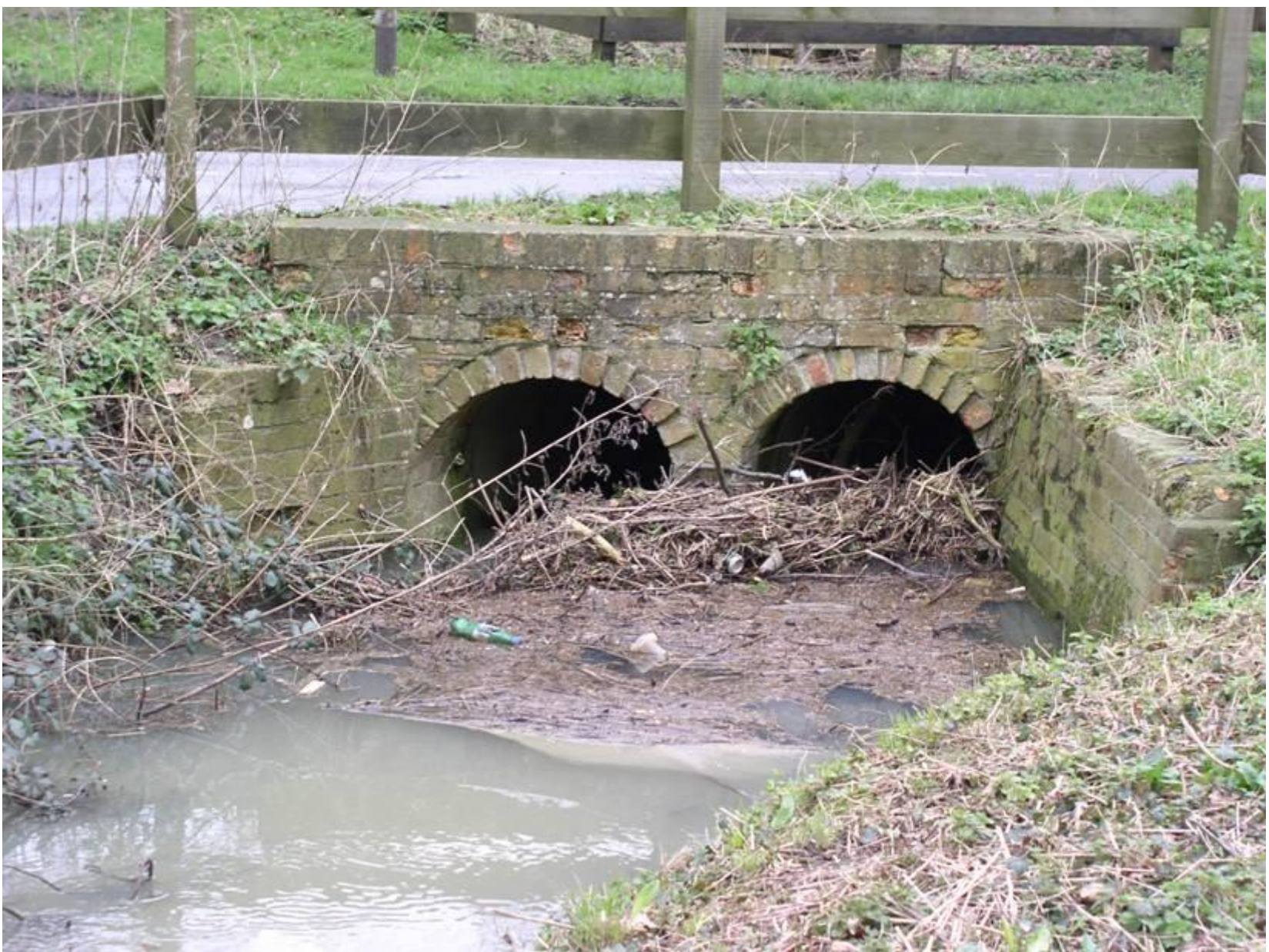
Build-up of natural debris + man-made items at the bridge in Brand's Pit between High Street and Fenstanton Road. This was causing some backing up of water.
