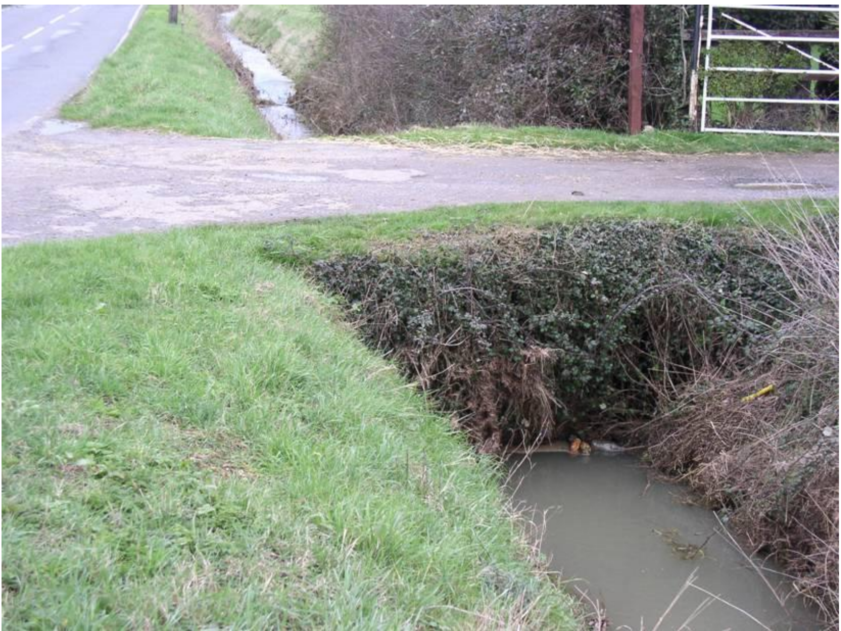
Build-up of natural debris + man-made items at the bridge to Hilton End Farm.
