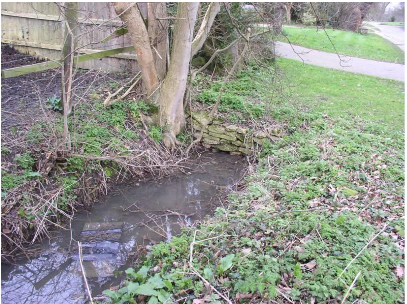
Water build-up at the culvert under the entrance to Sunnybrook.
