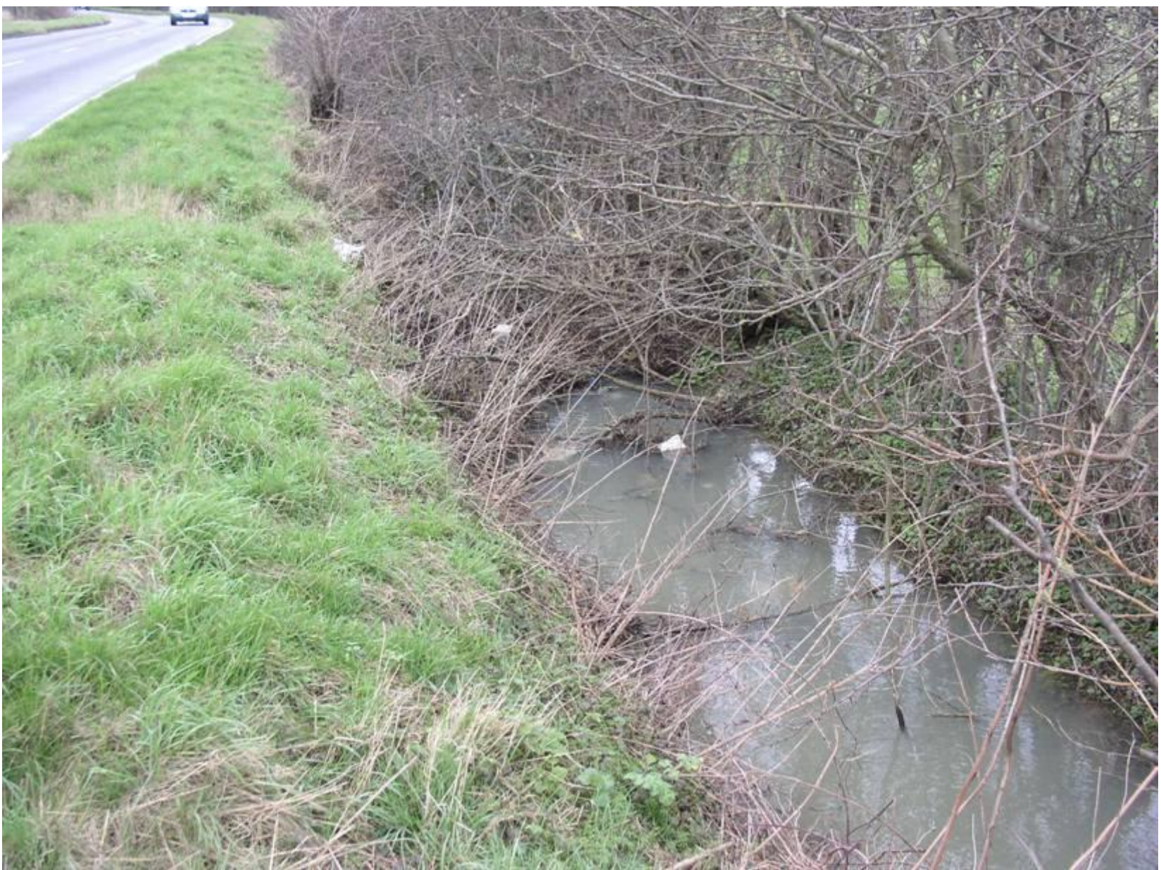
Build-up of natural debris + man-made items 200 metres north west of electricity sub-station entrance.
