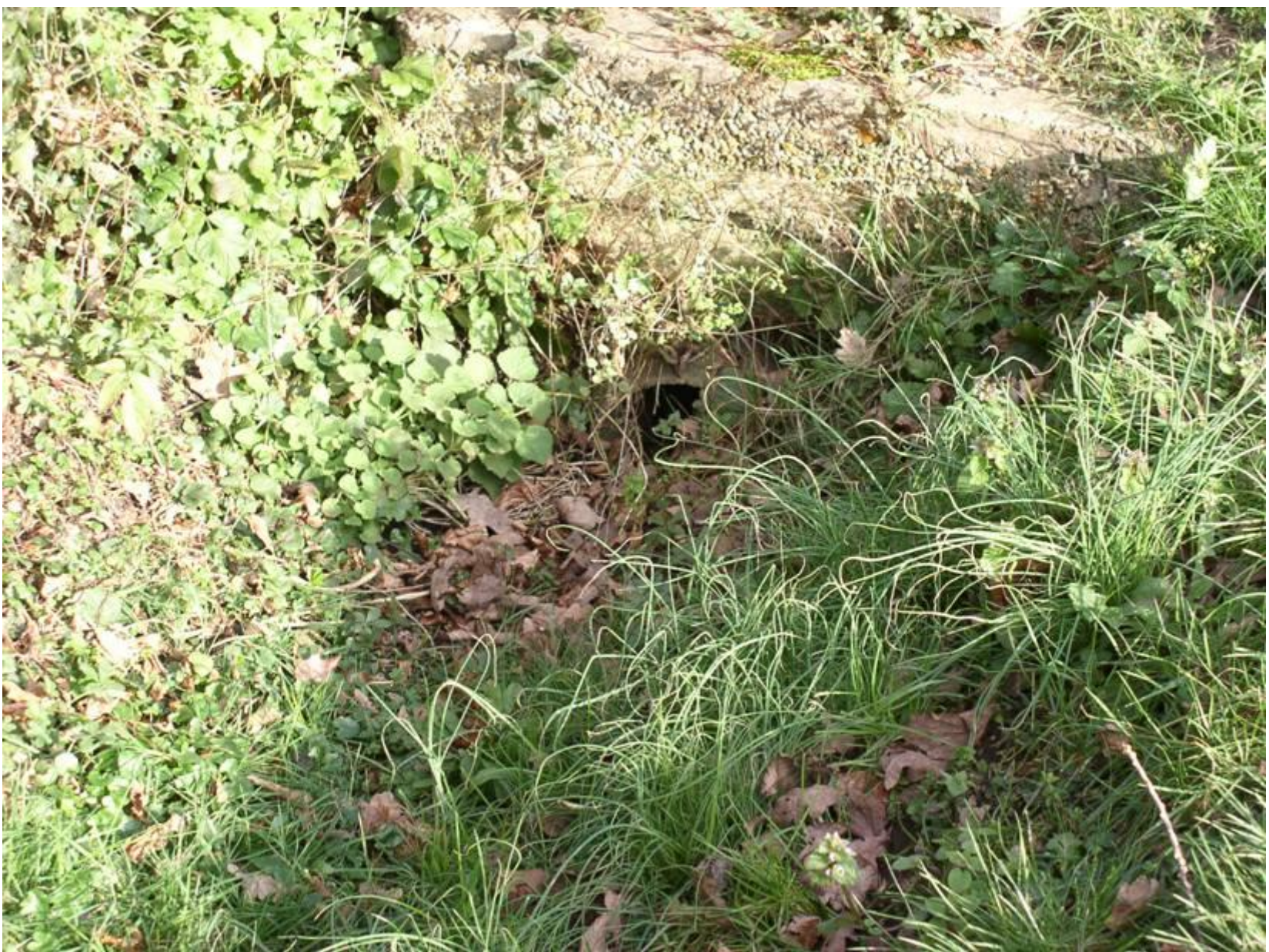
North-west end of the culvert for the entrance to Trin's Close. This shows that the ditch needs digging out.
