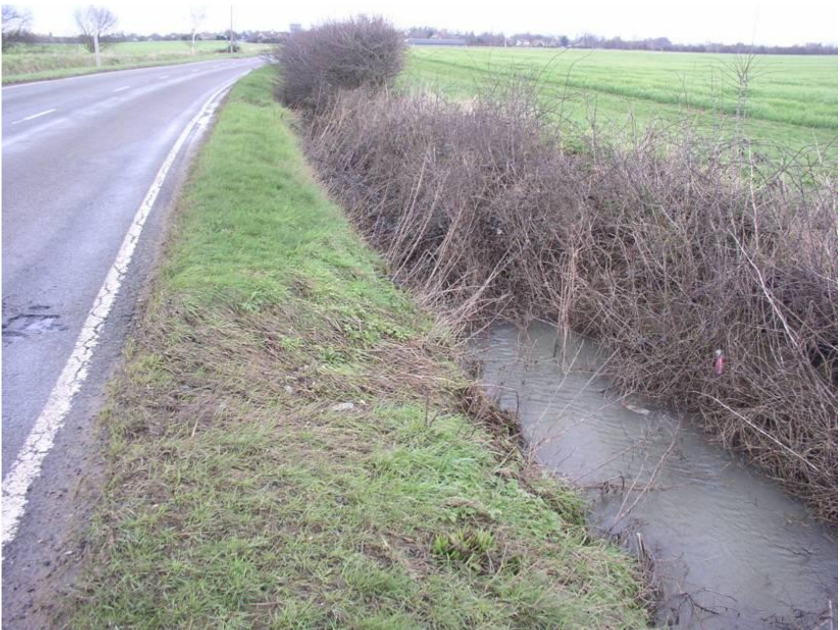
Weed growth over the ditch 75 metres north-west of New Farm.
