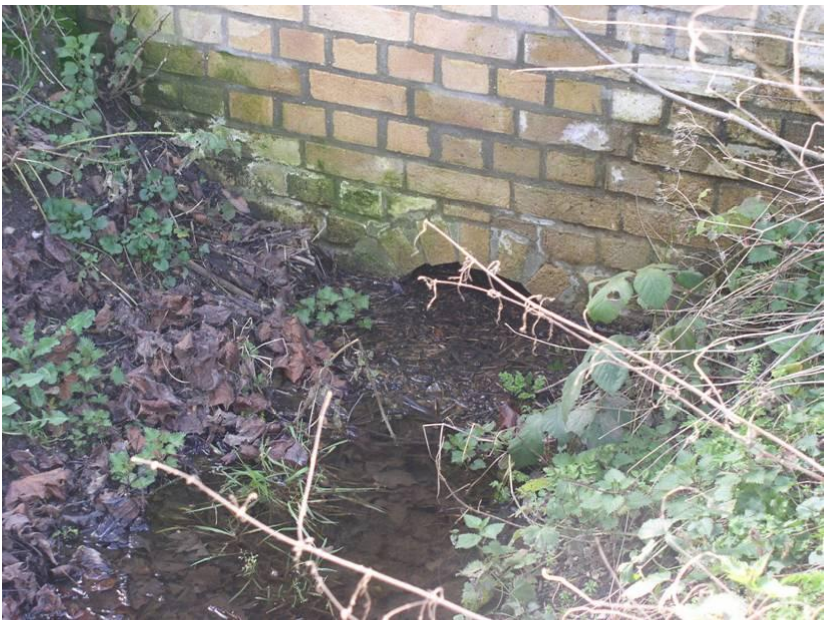
South-east end of the culvert for the entrance to Tarrant. Again this shows static water and again shows the need for the ditch to be dug out to allow water flow.
