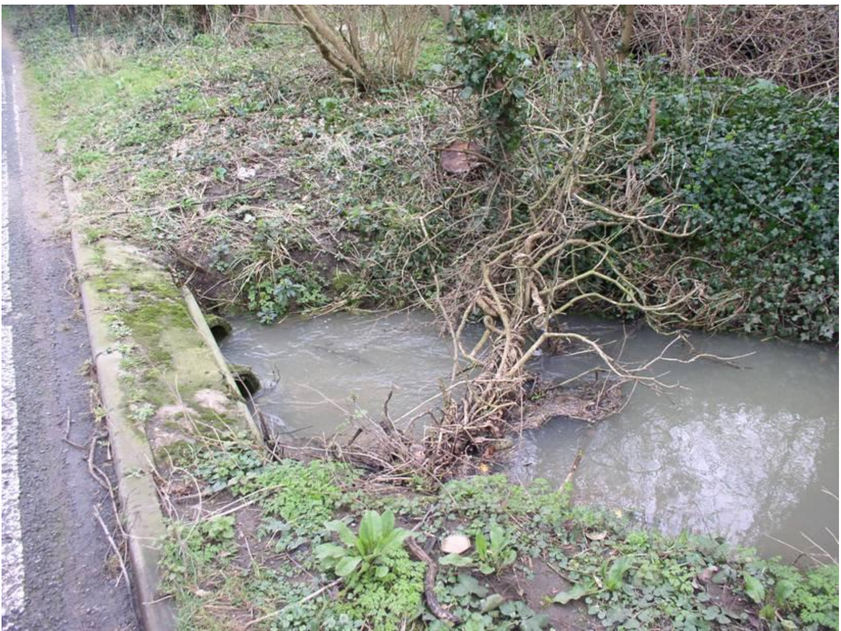
Build-up of natural debris at the 'occasional ford' in Church End.
