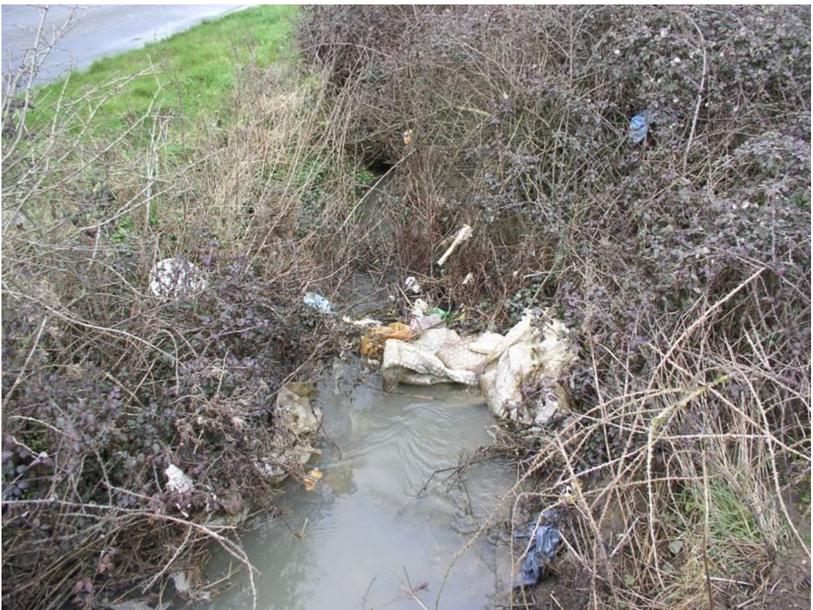
Potential blockage from discarded man-made items (plastic bottles and sheeting), at the electricity sub-station on the B1040.
