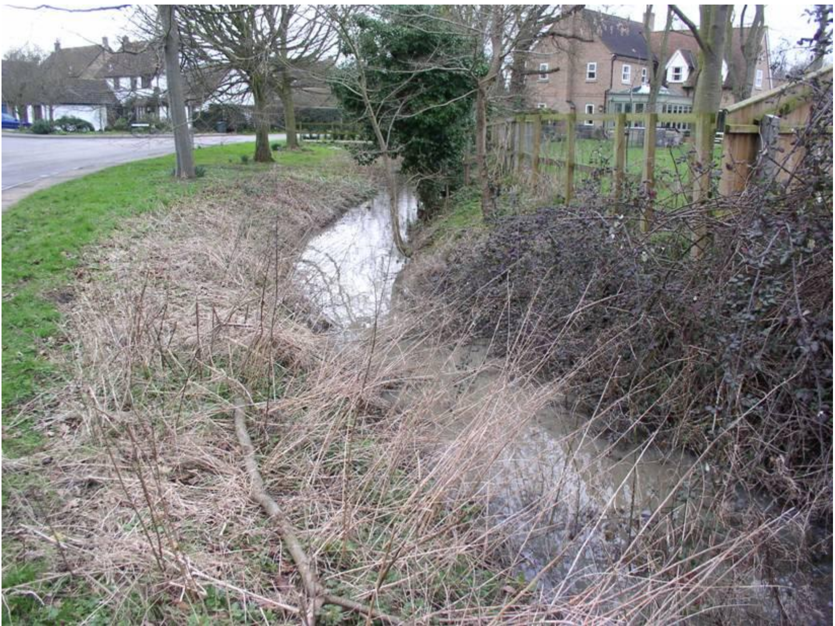
Standing water in the ditch at the North Western end of High Street.
